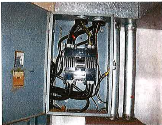
Typical Meter Room Main CB with Shunt Trip
