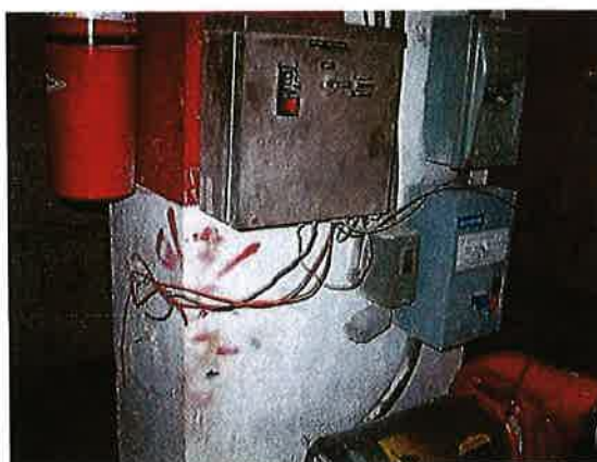
Open wires in pool room
