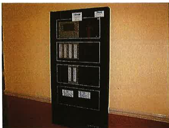
Fire Alarm Control Panel
