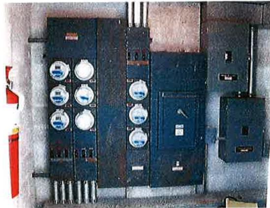
Typical Meter Room
