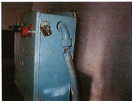
Broken Flex in trash room
