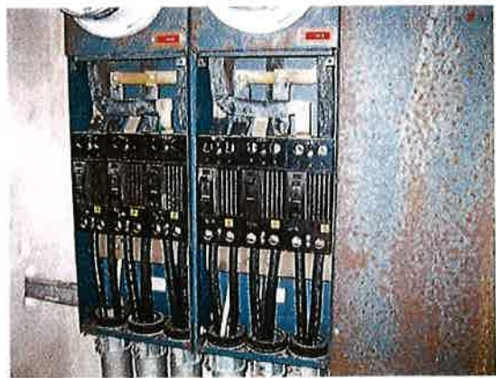
Typical Meter Room Apartment CBS
