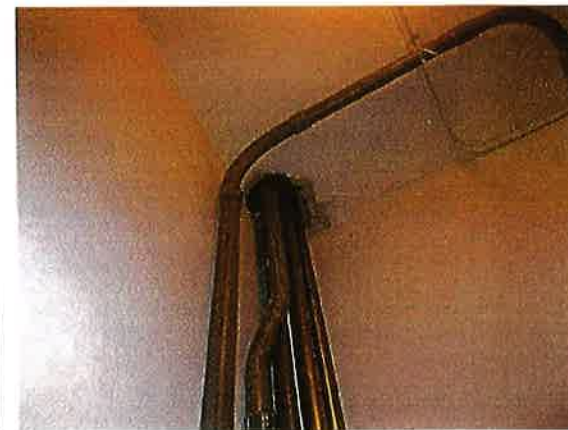
Typical Hole in Ceiling
