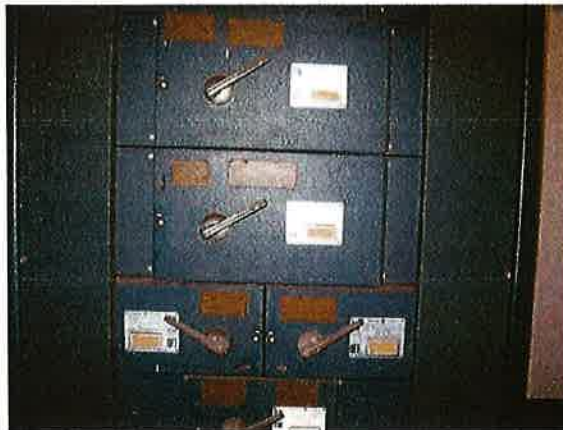
Main Switch Board Disconnect Switches
