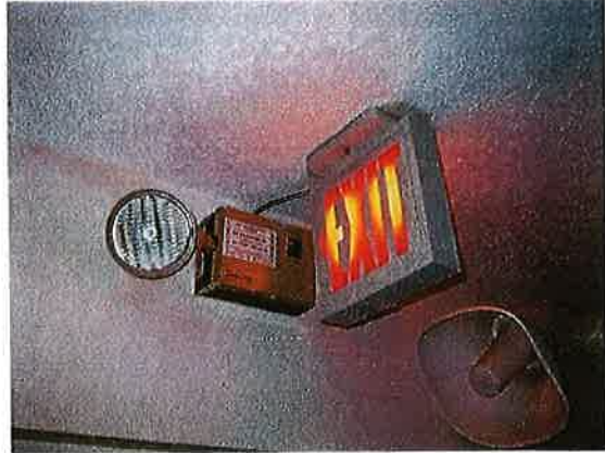
Exit sign and EM Light with Romex
