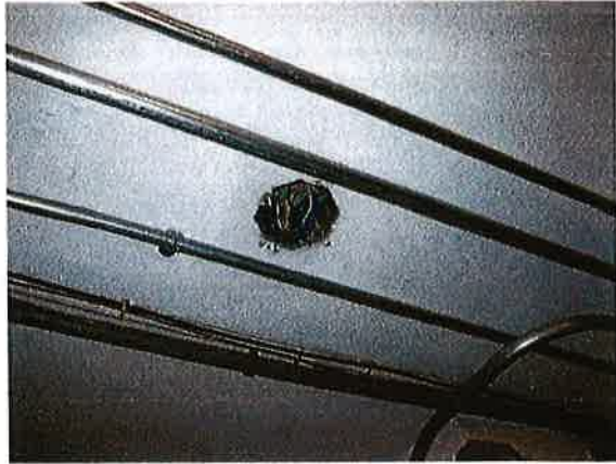
Open Junction Box
