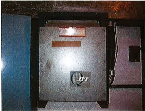
45 KVA Transformer with Main Electric Room
