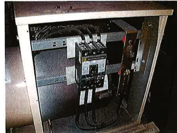
New Generator CB
