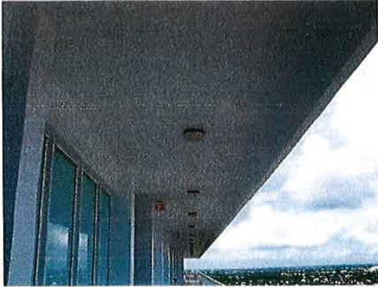
Outside lights require repairs
