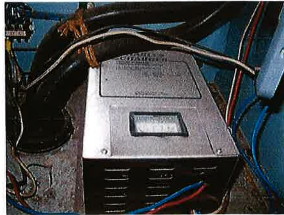
ATS with Battery Charger
