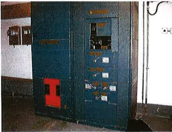
Main Switch Board
