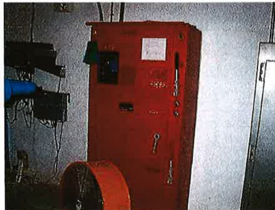
Fire Pump Controller
